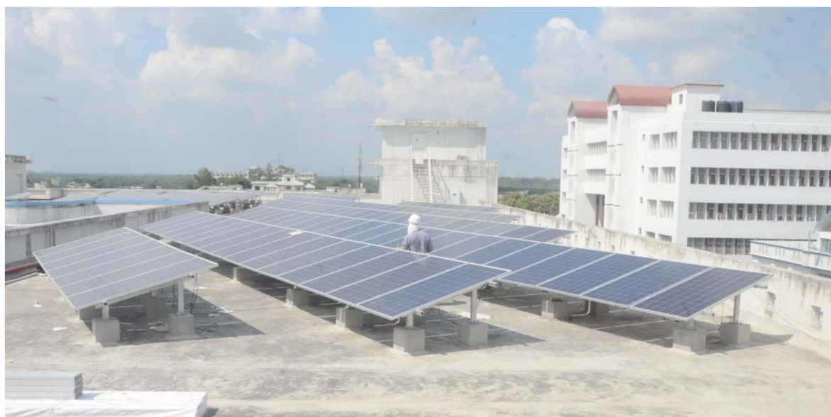
FIGURE 4 : Solar light installation on the terrace of Departments.
